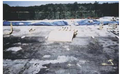
The hollow-core plank were shot-blasted and cleaned so they could be inspected for damage. Although some pieces were damaged, all appeared able to be reused.
